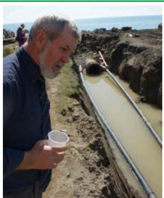
Kim Turnbull examines the intake pipe for the LADI Project
